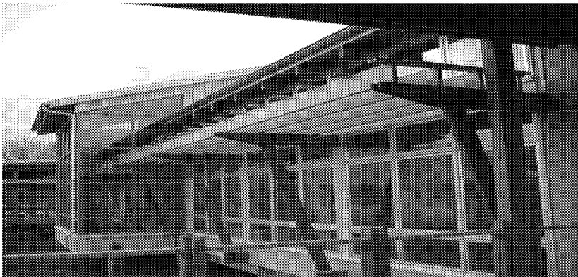
Window netting installed feet from window on slanted wooden beams. Photo by USFWS
