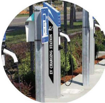
Electric Vehicle Charging Station
