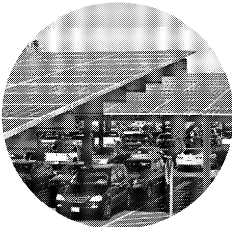
Roof Structure Solar Panels
