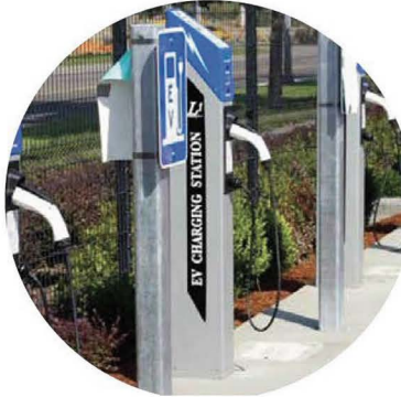
Electric Vehicle Charging Station
