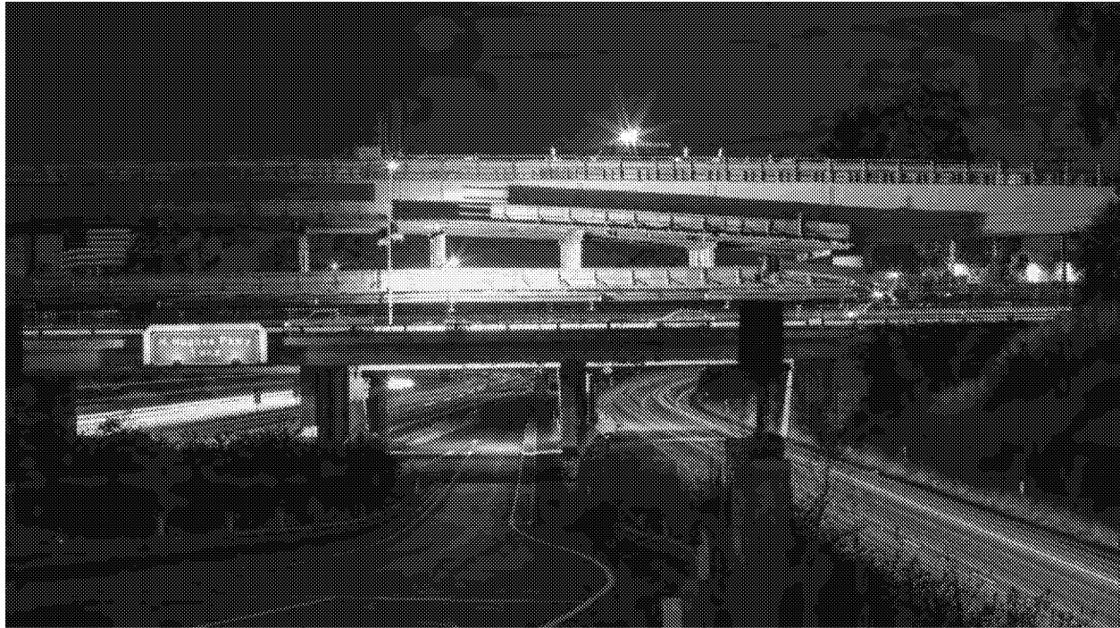
Construction crews work to complete a bridge for the Crenshaw Line along Florence Avenue in Inglewood in 2017. (Jay L. Clendenin / Los Angeles Times)
