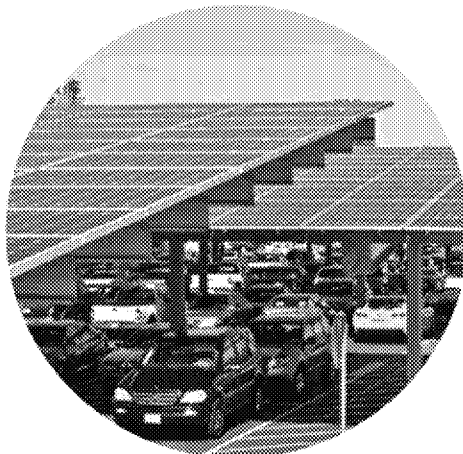
Roof Structure Solar Panels
