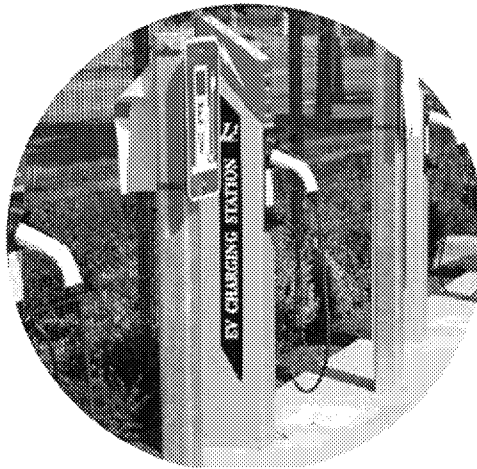
Electric Vehicle Charging Station
