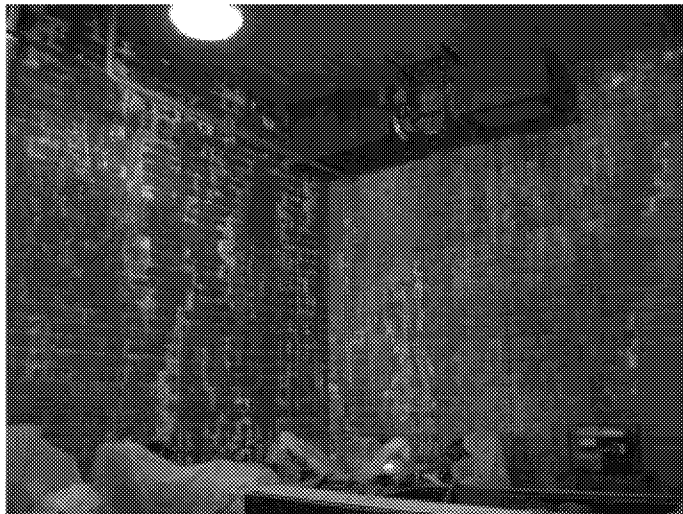
Figure 5.7 Moisture Effect on a Shear Wall
