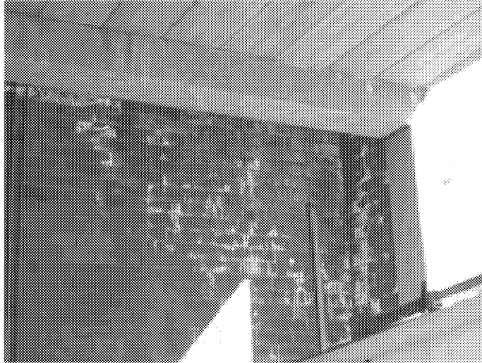
Figure 5.8 Moisture Effect on a Shear Wall
