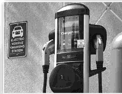
Level 2 charger at Walgreens
