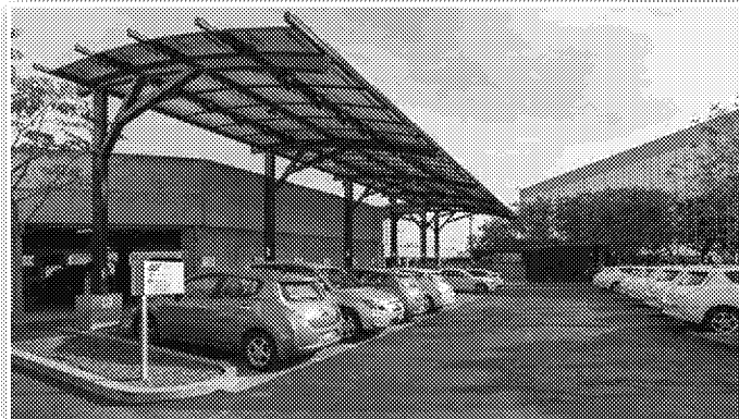
Employees and fleet operators charge their PEVs at San Diego Gas & Electric.
